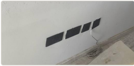
A19 SITE: living — existing socket run [OPN]
