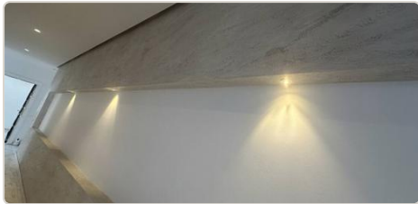
A25 SITE: main corridor — existing cove lighting [MCR]
