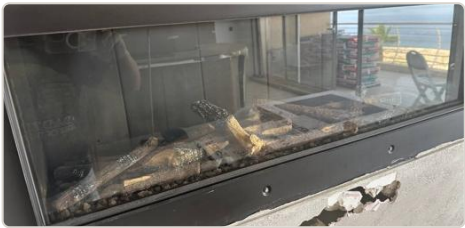
A18 SITE: fireplace close-up — installed, wall broken beneath [OPN]
